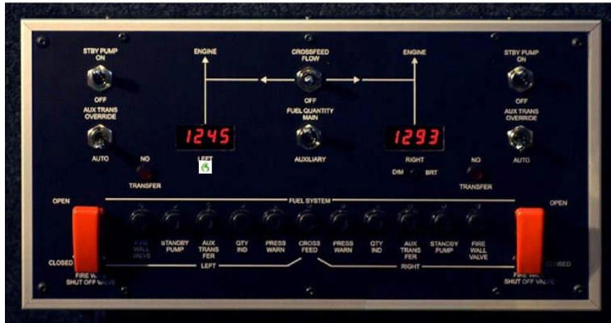
Fuel Side Control Panel
